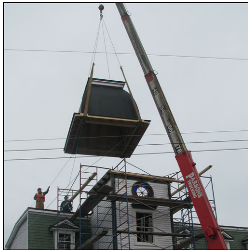
Installation of the Court House tower roof in 2010, returning it to its original architecture.
